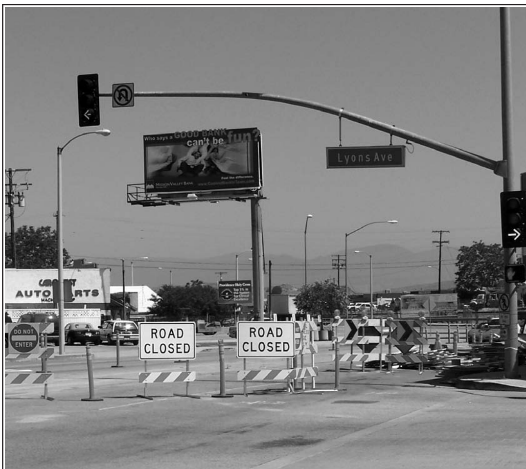
THE "ROAD CLOSED" SIGNS WHERE SAN FERNANDO ROAD NOW DEAD-ENDS AT LYONS AVENUE ARE ALSO SIGNS THAT THE REDEVELOPMENT OF OLD TOWN NEWHALL IS NO LONGER JUST AN IDEA – IT'S REALITY.
