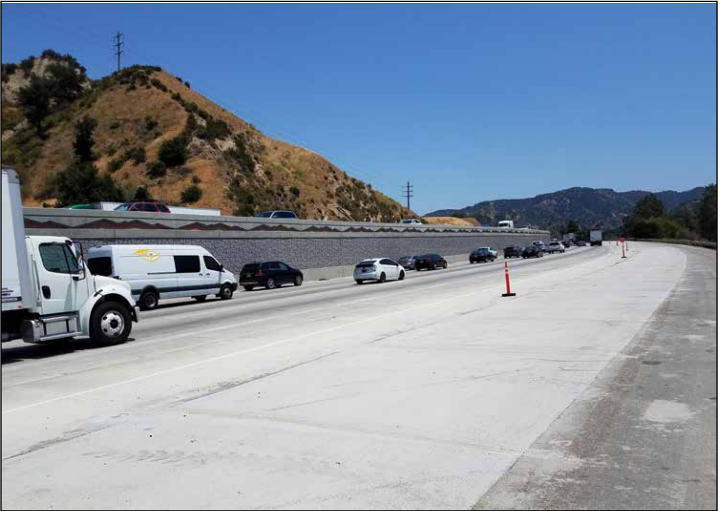
The Interstate 5 pavement rehabilitation project is making progress toward its 2019 completion. Shown in these photos: Newly repaved lanes nearing completion near Calgrove Boulevard. Photos courtesy of Caltrans
