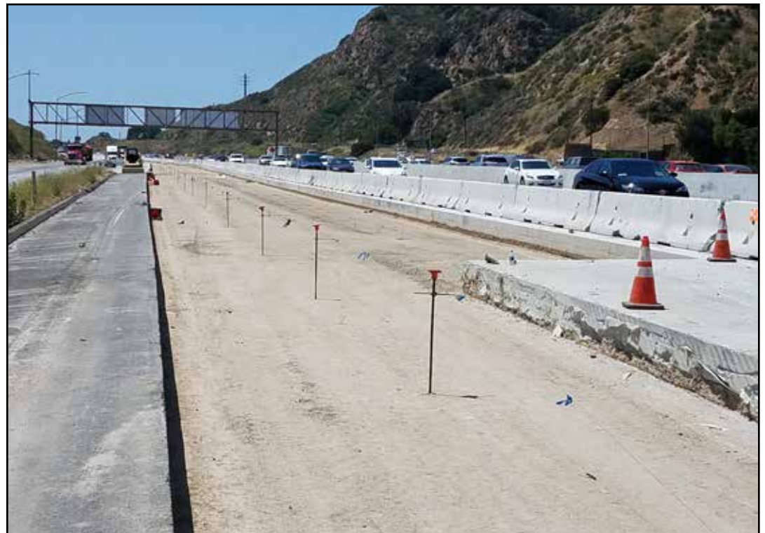
These lanes in the Newhall Pass are shown after being fully excavated in preparation for the new pavement. Photo courtesy of Caltrans
